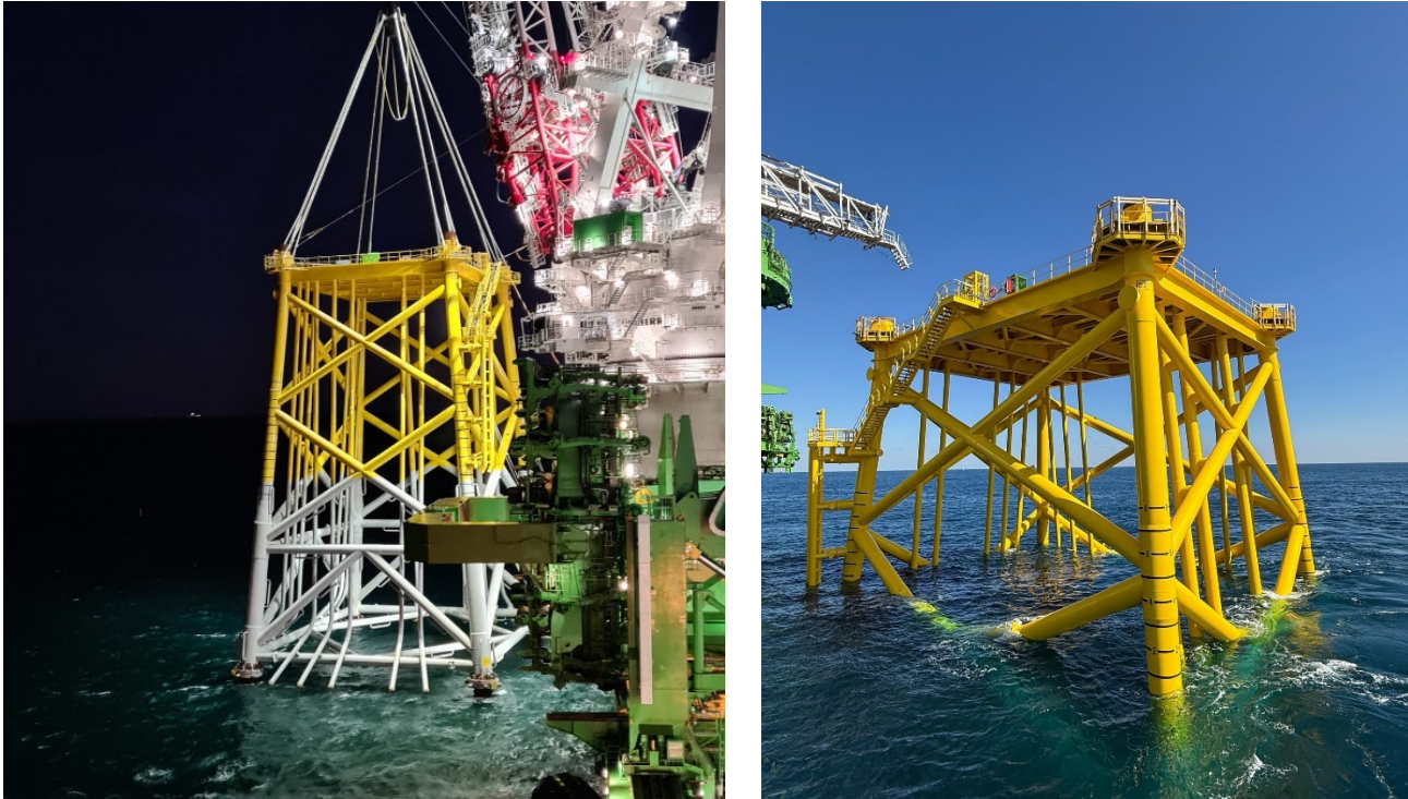
Offshore Substation being lowered to the seabed and the OSS fully submerged
