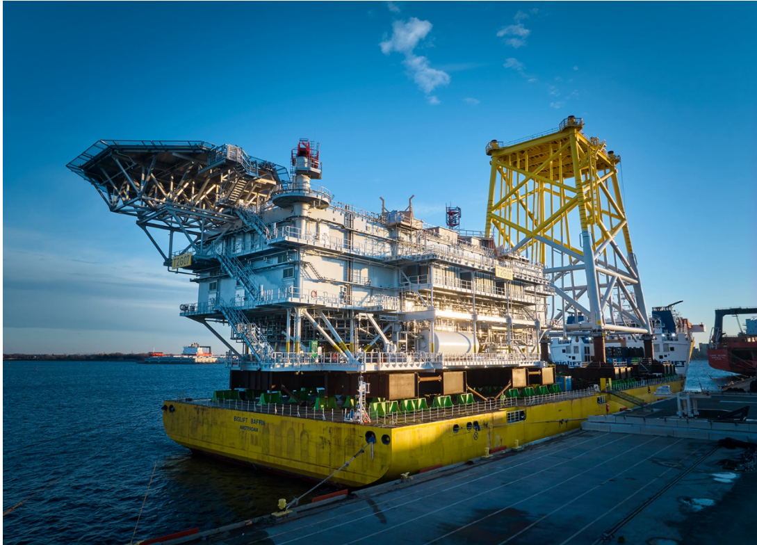
BIGLIFT BAFFIN loaded with the jacket foundation and topside for Offshore Substation (OSS) #2.
