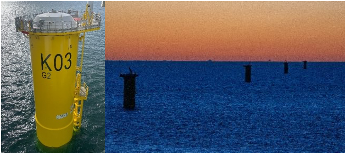
Figure 7: Temporary marine navigation lights on installed TPs
