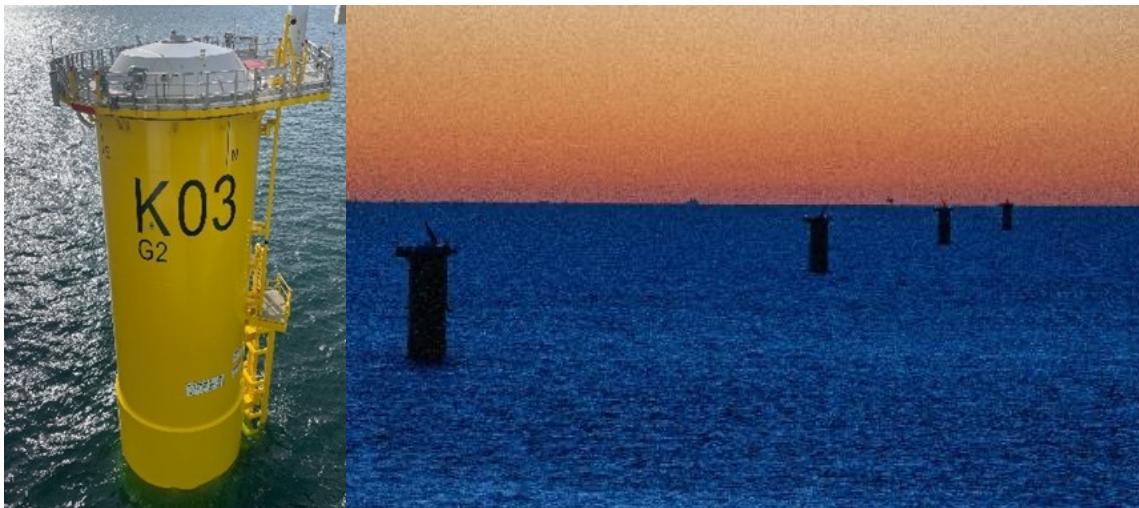
Figure 7: Temporary marine navigation lights on installed TPs
