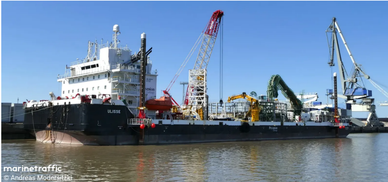
Figure 6: Cable Lay Barge ULISSE will be supporting cable landing and shallow water cable installation
