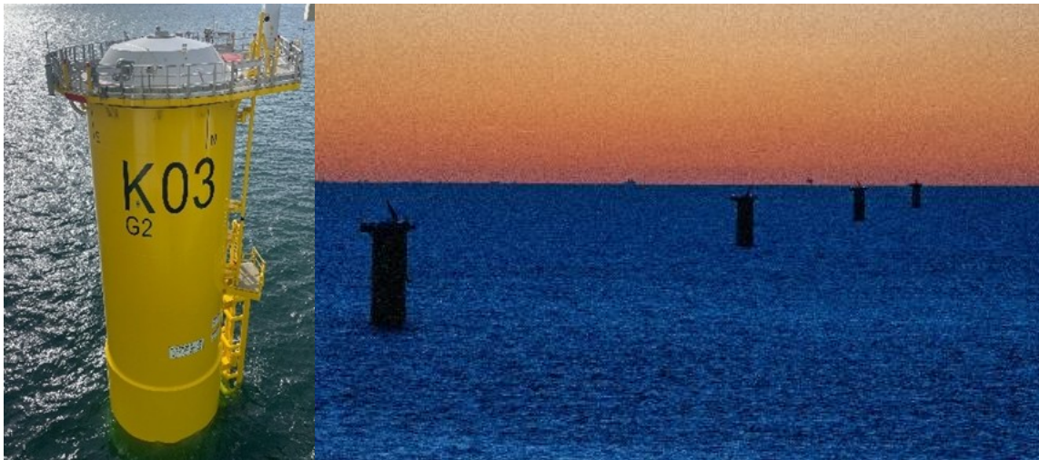
Figure 10: Temporary marine navigation lights on installed TPs
