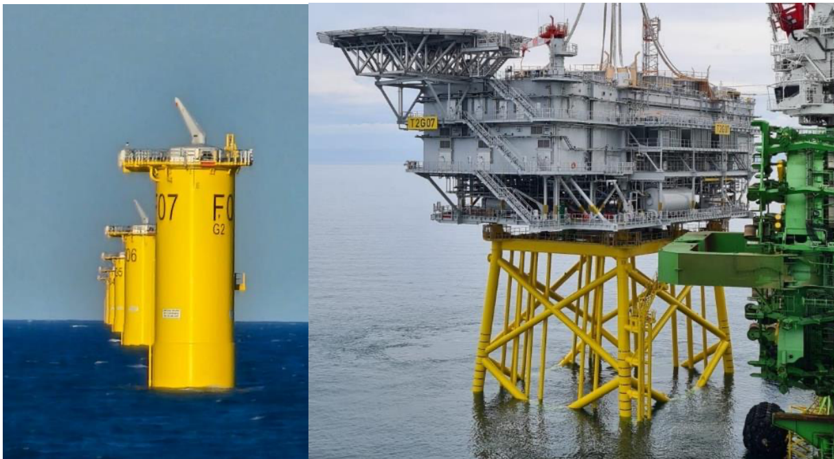
Figure 5: Installed TPs along "Row F" spaced 0.9-miles apart and Offshore Substation with Topside.
