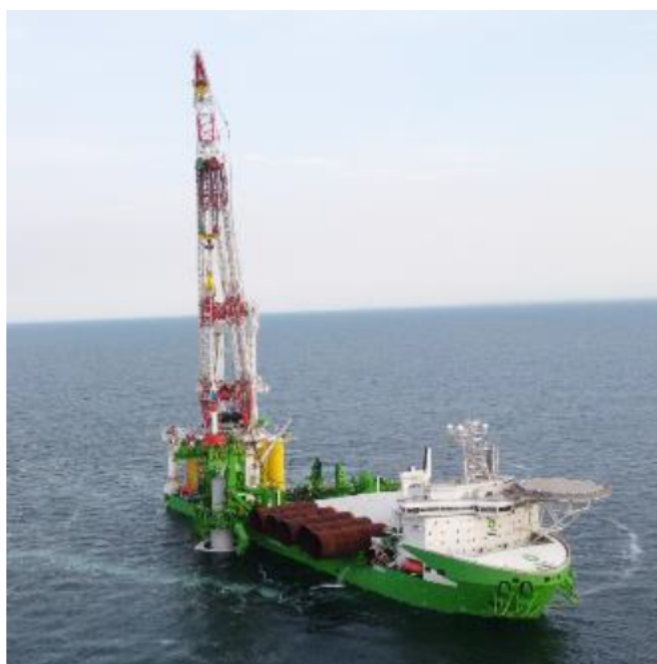
Figure 5. Aerial picture showing the placement of the hydro hammer on a MP at safe depth in the gripper of the installation vessel Orion on the Vineyard Wind 1 Project.
